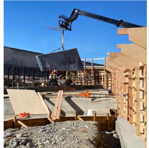
Construction at Mill Creek will allow sediment in diverted water to make its way back into the creek, limiting maintenance needs and returning the area to more natural conditions. Photo Credit: SBVWCD.
